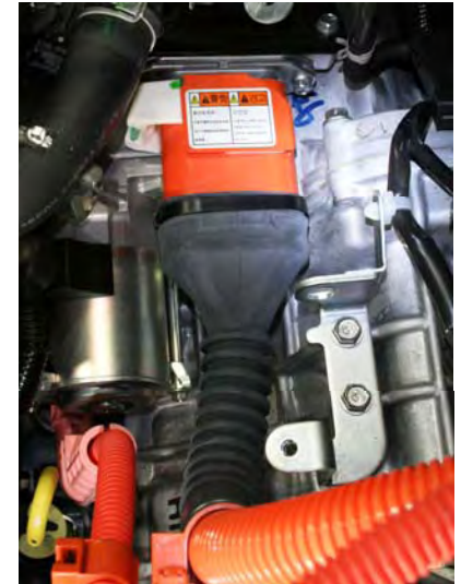
High-Voltage Cable Connection to Motor
